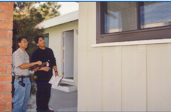
Gordon Hom and Nick Diaz, members of the construction management staff, visit a job site to make sure that all sound insulation products have been properly installed in a triplex on West Century Blvd.
